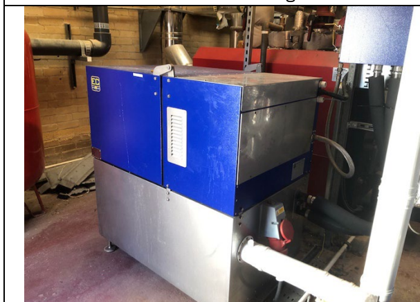
Non operational CHP
