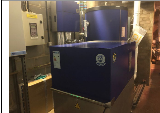
Non operational CHP
