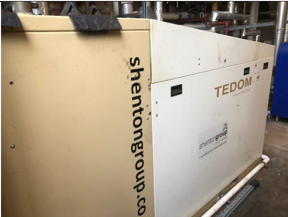
Non operational CHP
