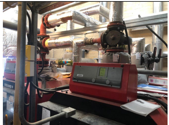
Boiler and uninsulated valve
