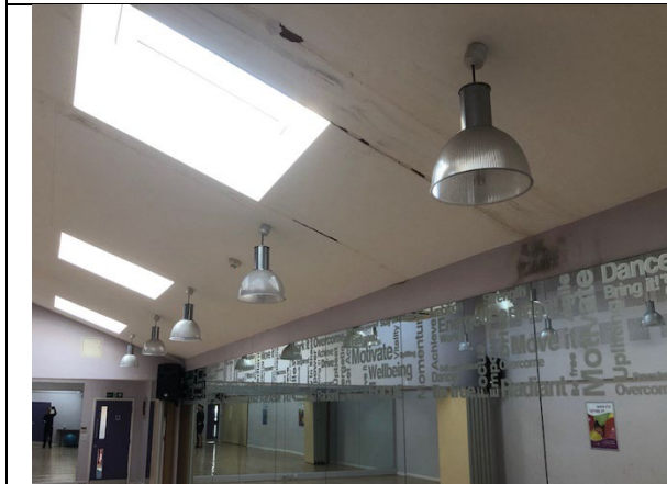
Gym lighting to be replaced
