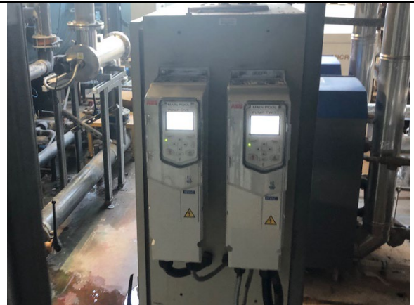
Circulating Pumps Inverter Control
